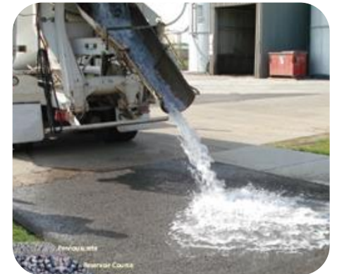
Instant Water Logging Solution
